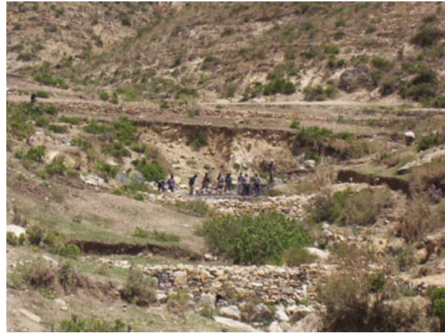
Figure 5. Partial view of the managed May Zeg-Zeg catchment, with check dams in the gully, exclosure at the back and stone bunds in farmland and in the exclosure
